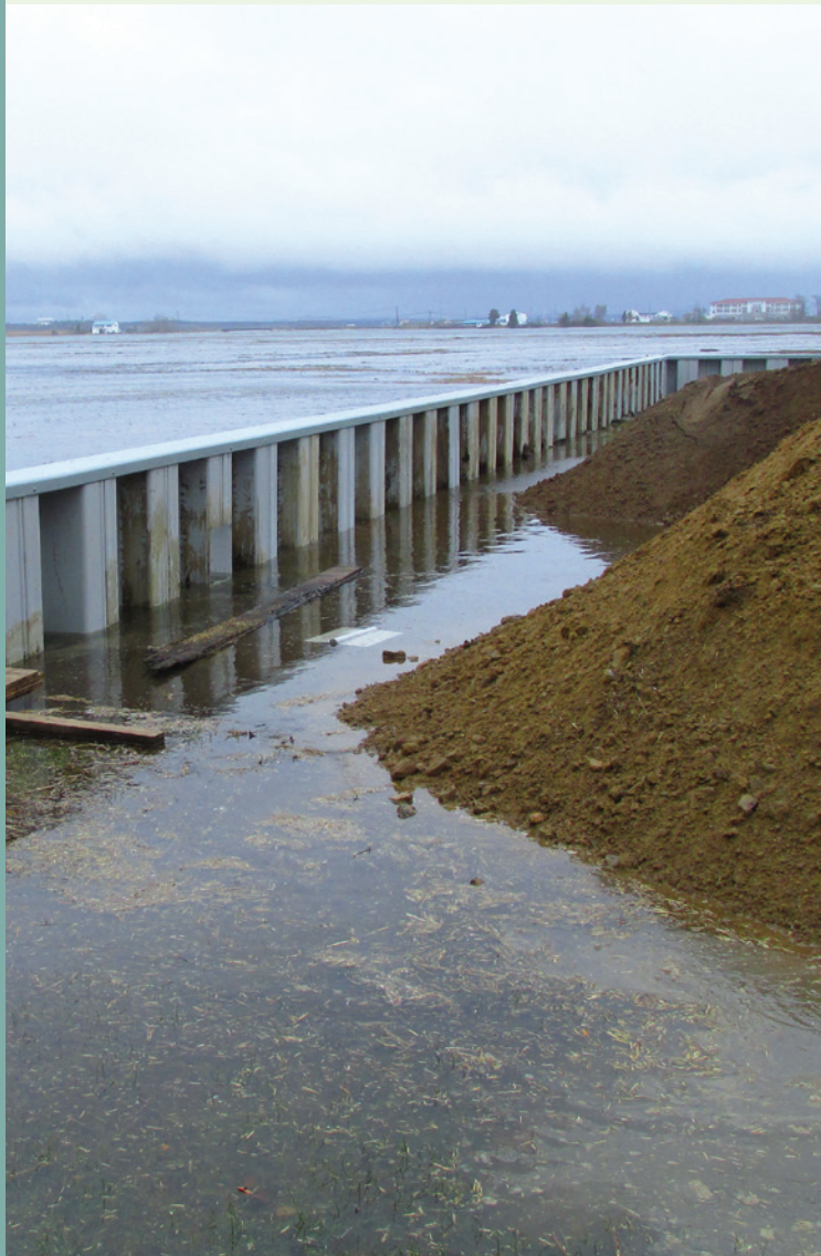
Flooded privately owned seawall along Northeast Massachusetts coast. Photo: Joe Teixeira, Newburyport, MA.
